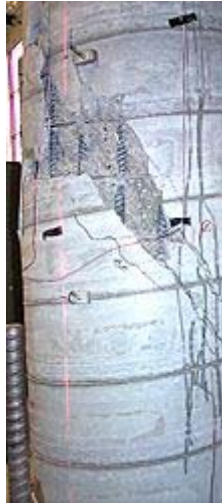
Photo: 1 Failed Column
